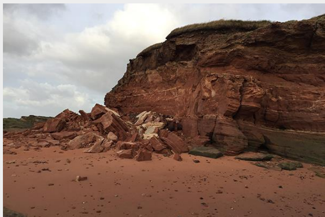
Rock fall at South End of Hilbre (January 2016)
